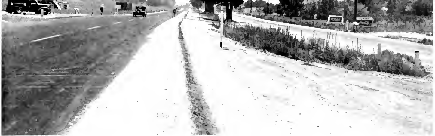
Four-lane divided highway East of Redlands. New construction for dual West bound traffic lanes on left. Existing highway on right
